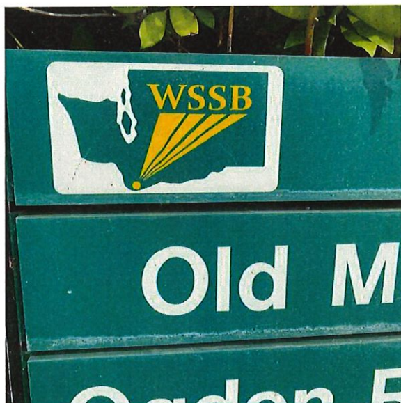
Old Main Signage with water deposits
