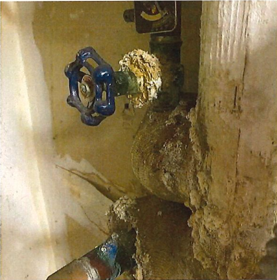
Typical valve on domestic hot water line
