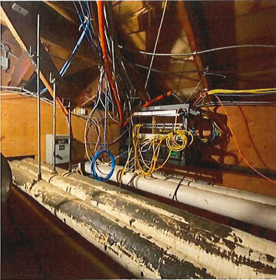
Communications equipment in unconditioned spaces
