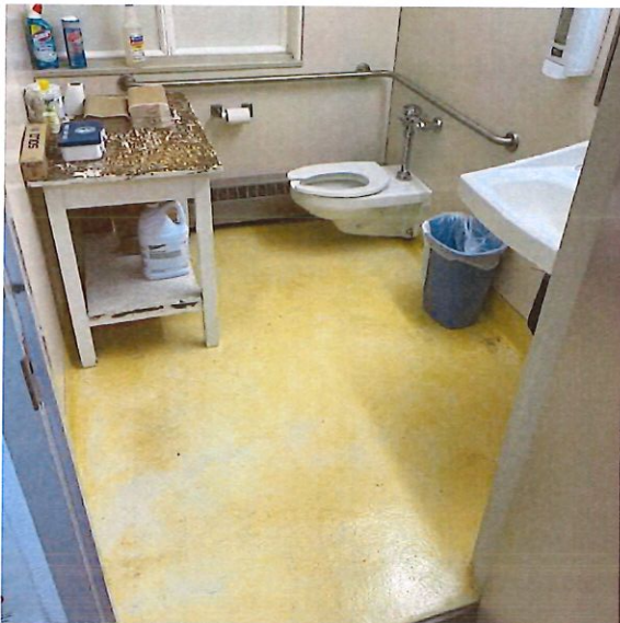
Dormitory 2 Staff restroom, floors shot
