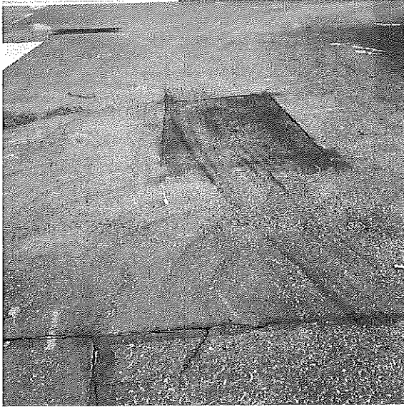
Old Main Parking Cold patch deformation and old sealer failing
