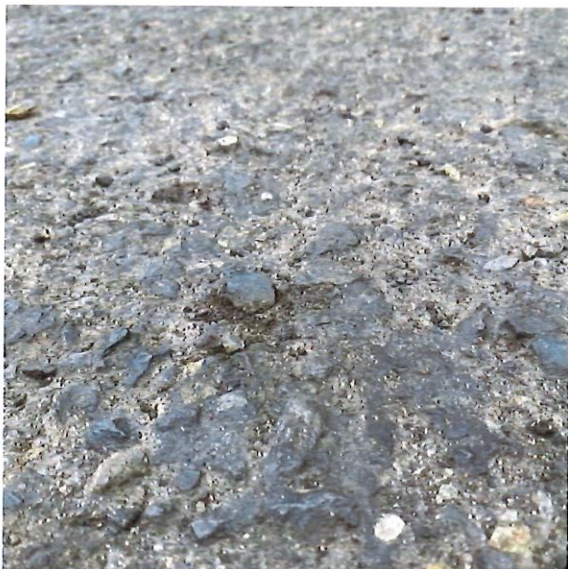
Old Main Parking Old sealer failing
