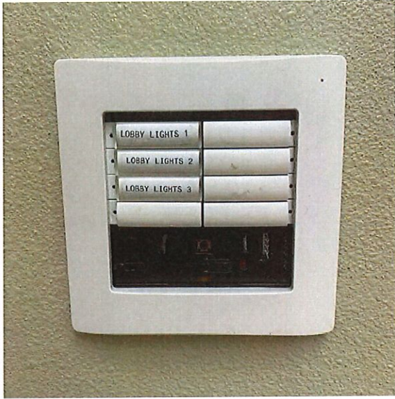
Stenehjem Fitness Center Typical light switches
