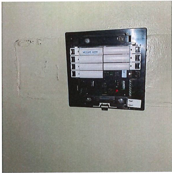
Stenehjem Fitness Center Typical light switches
