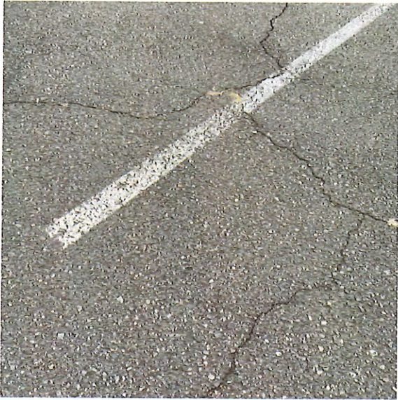
Gymnasium Parking Cracks prevalent
