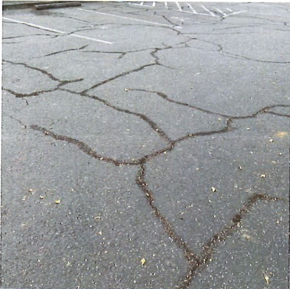
Childcare Parking Old seals failing
