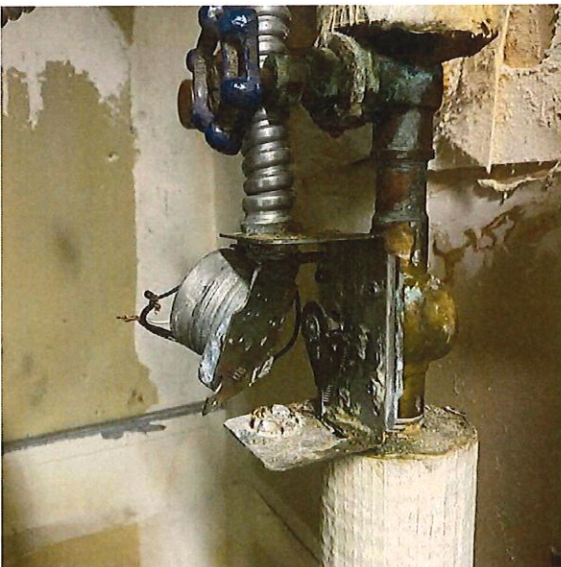
All heating loop zone valves need replacing
