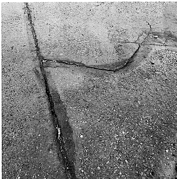
Old Main parking Cracks with vegetation
