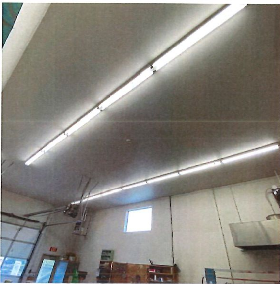
Maintenance Building Fluorescent Lighting
