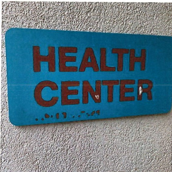
Old Main North Health Center Entry Braille deteriorated, unreadable
