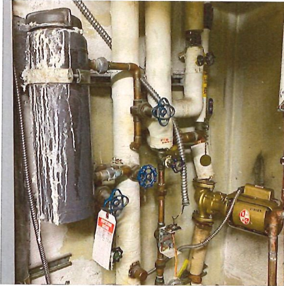
Dormitory 3 Loop chemical treatment tank
