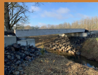
Removing fish barriers and replacing them with bridges that allow fish access.
