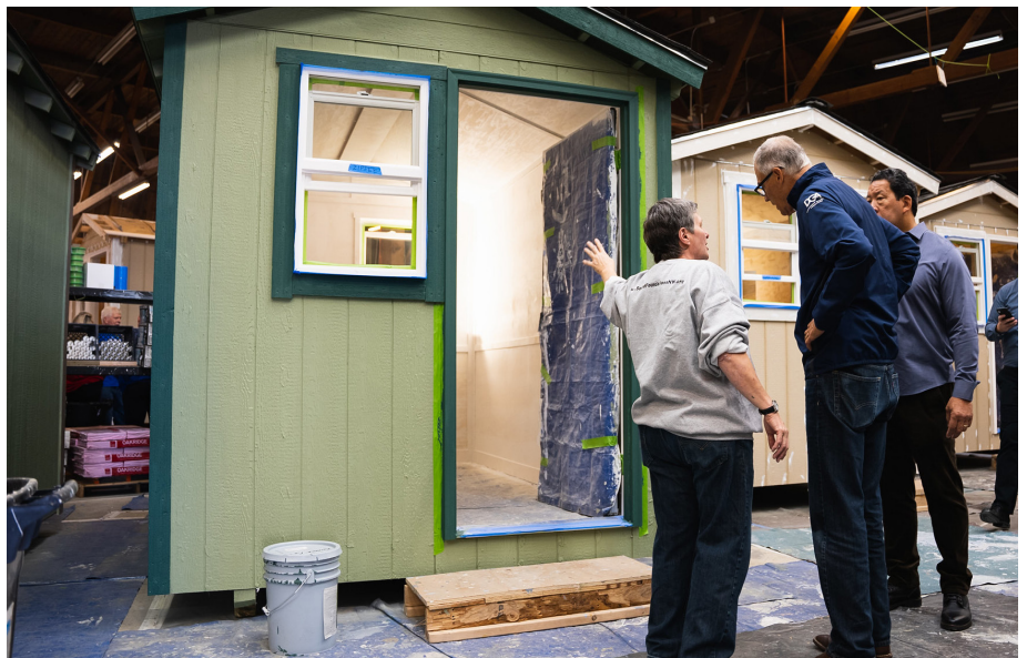
Sound Foundations NW builds tiny homes at its 'Hope Factory' with volunteer labor. Gov. Jay Inslee and Seattle Mayor Bruce Harrell take lessons from Sound Foundations NW Director Barb Oliver before they help build a tiny home. (Office of the Governor photo, October 2022)
