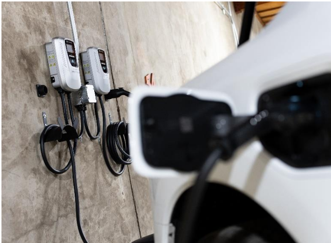
These EV chargers at the Cowlitz Indian Tribe Transportation Center are powered by solar panels and funded in part by the CCA.
