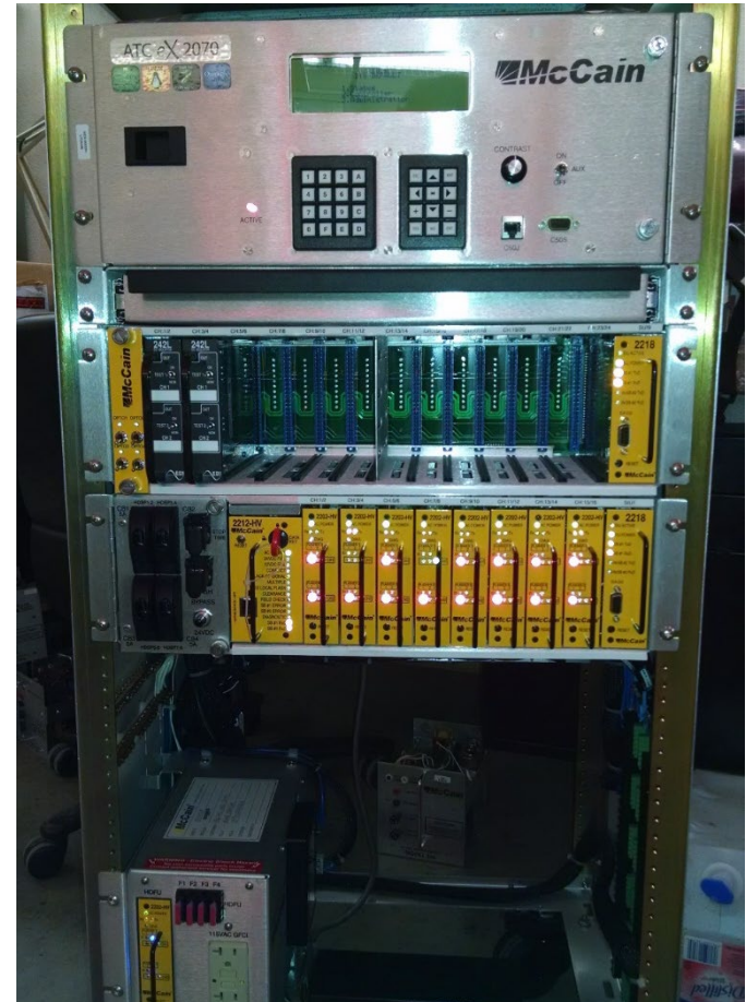
Advanced Traffic Control (ATC) Cabinet • Shift from 40-yr legacy
