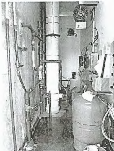
Looking into WTP control room
