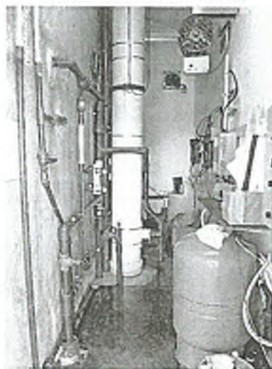
Looking into WTP control room
