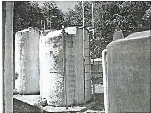
Contact tanks, left and right; equalization tank, center
