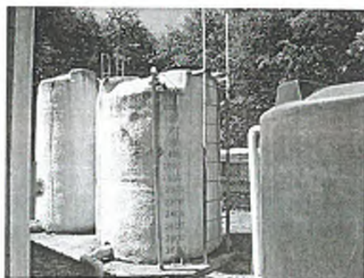
Contact tanks, left and right; equalization tank, center
